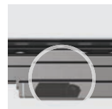
DMX power supply units inside the body of the luminaire
